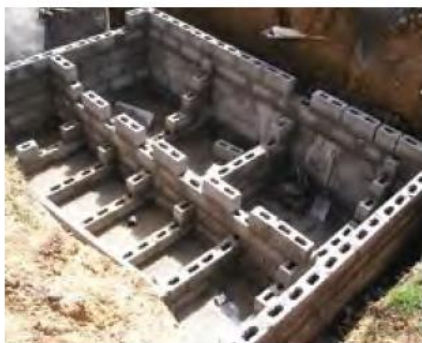
Picture 34: Anaerobic baffled reactor under
